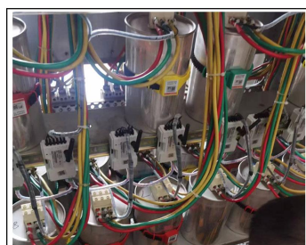
Switchboard Temperature Monitoring Point Showcase
