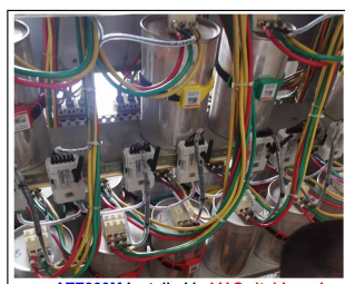
Switchboard Temperature Monitoring Point Showcase
