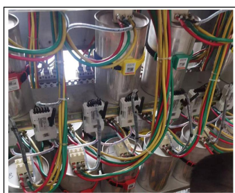
Switchboard Temperature Monitoring Point Showcase
